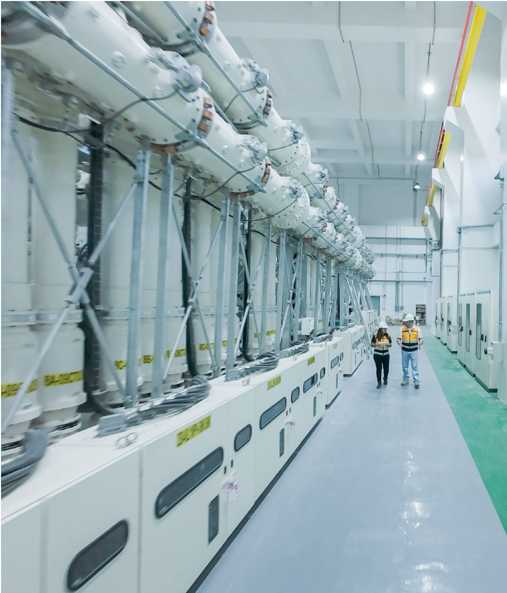
In our 585 MW SanMar Solar, we built a gas-insulated type substation with intricate engineering requirements to accommodate large amounts of renewable generation.
