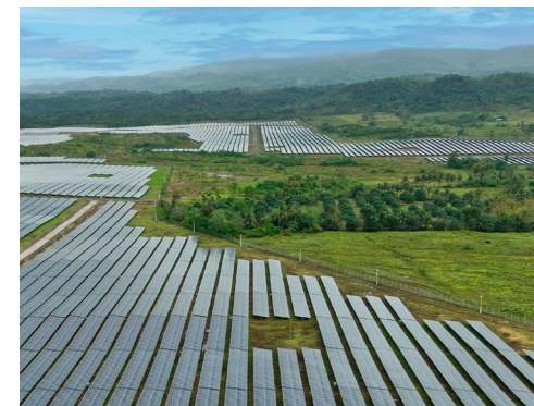
The 133 MW Cagayan North Solar is the first utility-scale solar in the Cagayan province.
