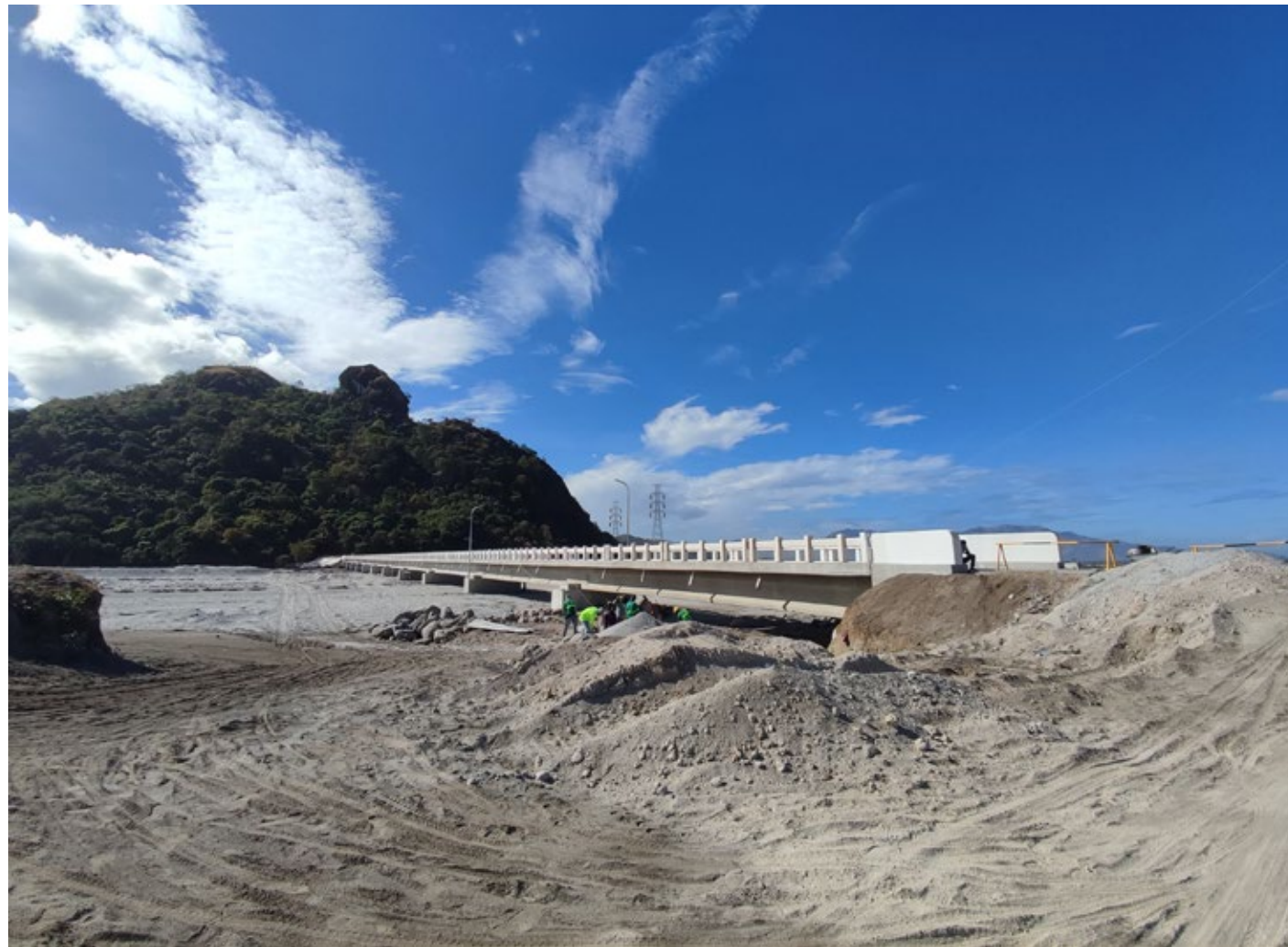
A 330 meter concrete bridge that we built for communities surrounding our 283 MW SanMar Solar project in Zambales, Philippines now allows the locals to pass through without wading in lahar.
