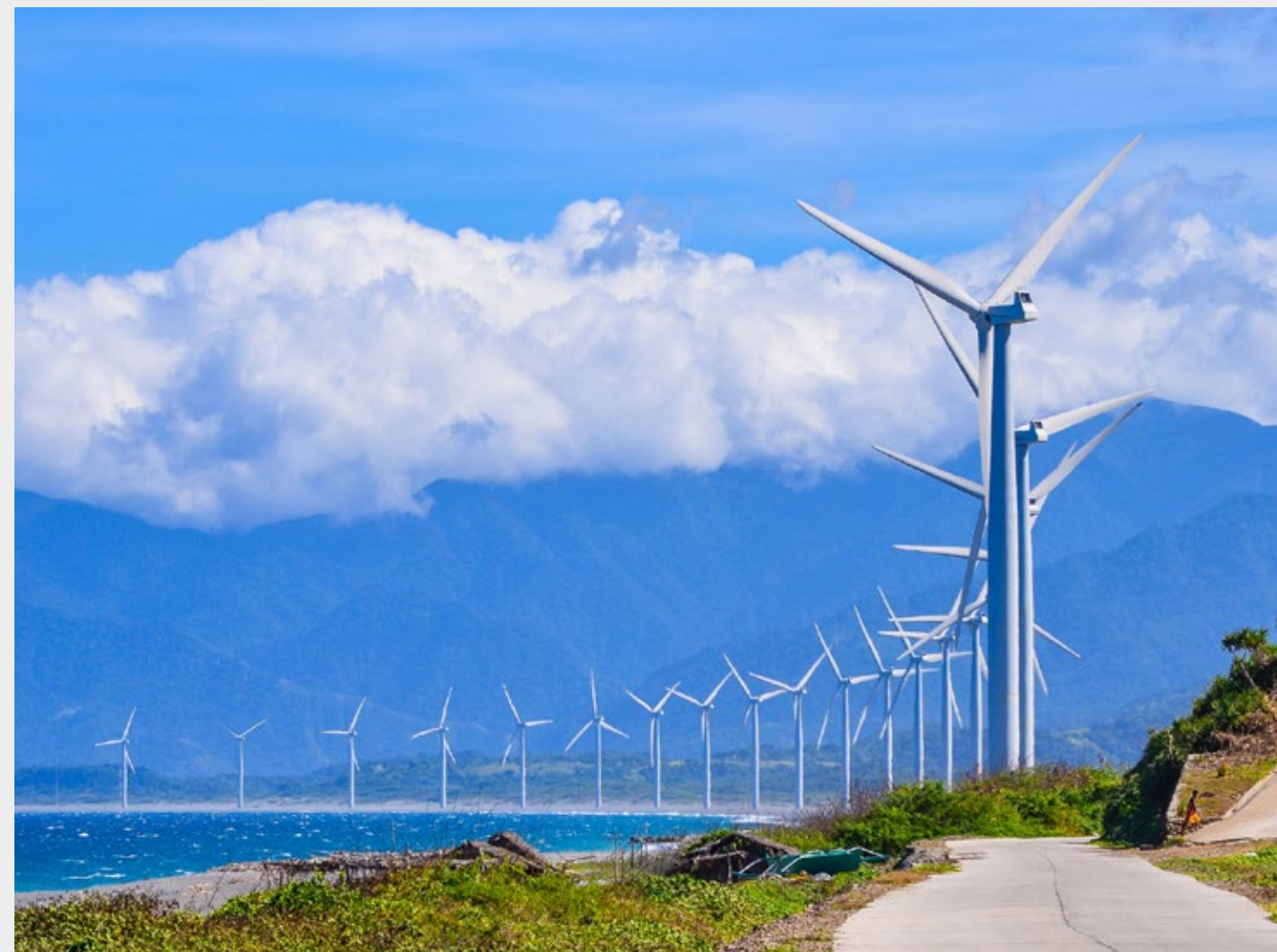
ACEN's 52 MW NorthWind in Bangui, Ilocos Norte is Southeast Asia's first utility scale wind farm.
