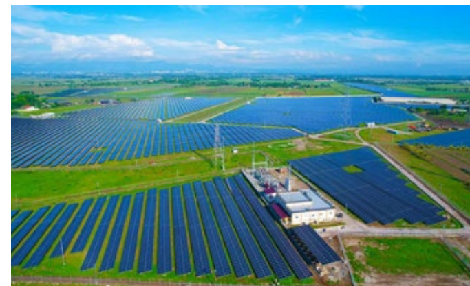
The 72 MW first phase of the Arayat-Mexico Solar Farm, a joint venture between ACEN and Citicore, started operations in 2022. It is expected to generate 105 GWh of renewable energy annually, which can power approximately 45,000 homes.
